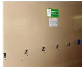
Photo of the sanitary facilities Drinking water point.JPG
