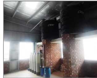
Photo of the inside of the main production hall Water purifier.JPG
