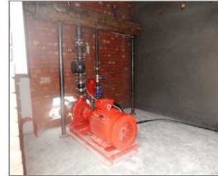
Photo of the inside of the main production hall Jockey pump.JPG
