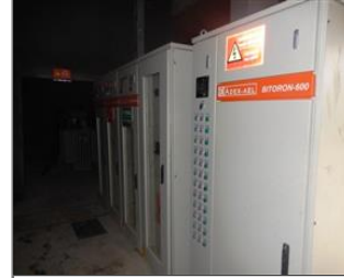
Photo of the inside of the main production hall Switchgear.JPG
