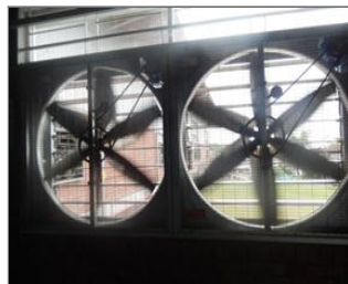
Photo of the inside of the main production hall Exhaust fan.JPG
