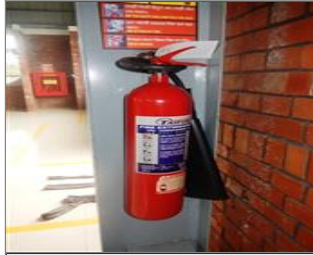
Photo of the inside of the main production hall Fire extinguisher.JPG
